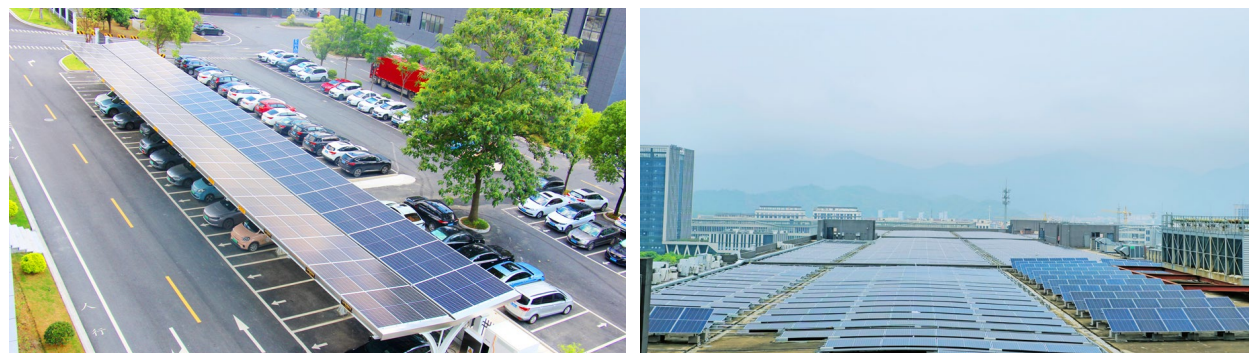
Rooftop PV and PV Charging Carport
